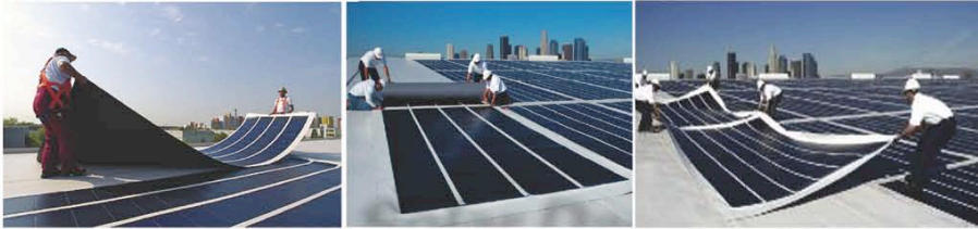
active use of solar energy: flexible photovoltaic cells
